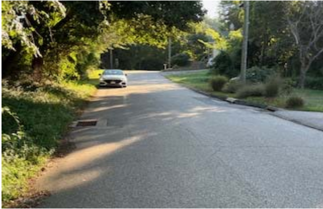
Catch basin on Cedar Lane
