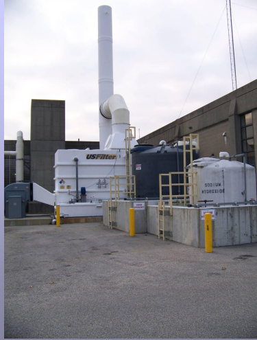
Odor control at the headworks
