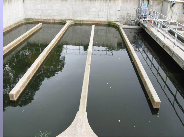
Chlorine contact tanks
