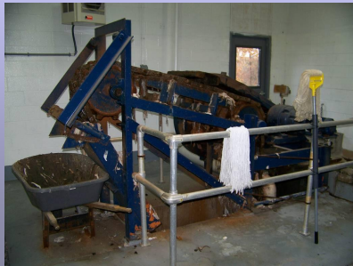
Catenary bar screen
