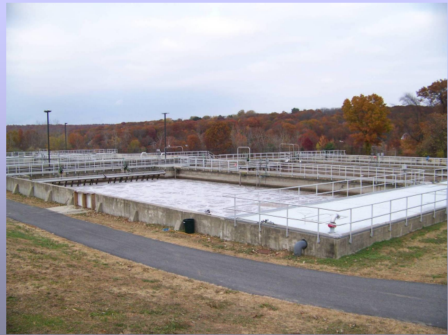
Sequencing batch reactor (SBR) basin
