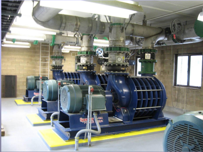
Sequencing batch reactor (SBR) blowers
